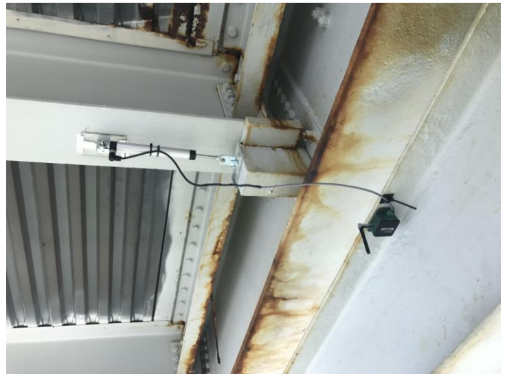
Resensys Wireless Displacement SenSpot™ sensor for monitoring bridge under superloads
