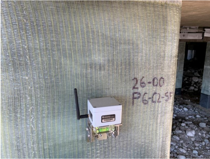
Resensys Wireless Tilt/Inclination SenSpot™ sensor on pier for monitoring bridge under superloads
