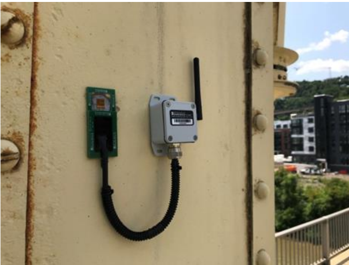
Resensys Wireless Strain SenSpot™ sensor for monitoring bridge under superloads
