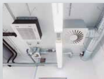
Noise generated by HVAC systems
